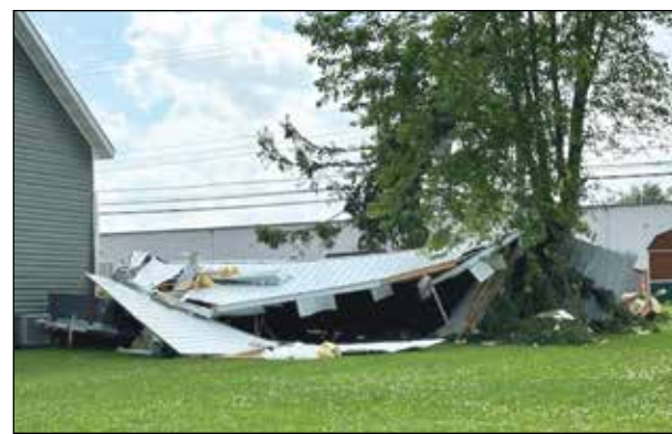
Six low-grade tornadoes in the Colby area this spring and early summer have caused significant storm damage the past few months.
