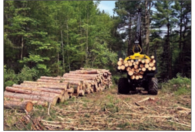
The initial clearing of the three-plus acre parcel took place recently. The plan is to have 16 homes and a community center completed by the end of 2026.
