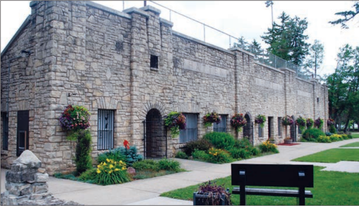
Hatten Stadium in New London dates back to 1935. The project was part of President Franklin D. Roosevelt's New Deal Work Progress Administration to provide employment to Americans during the Great Depression.
