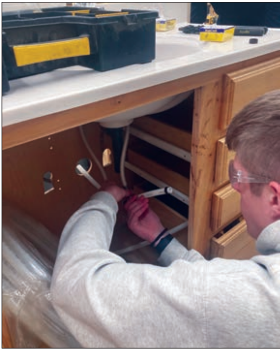
THS students learning plumbing skills Building Trades students at Tomahawk High School (THS) are learning plumbing skills, including how to run PEX tubing through a stud wall, connect fittings and install a trap for a vanity.
