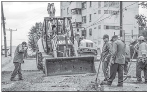
Use extra caution in work zones.
