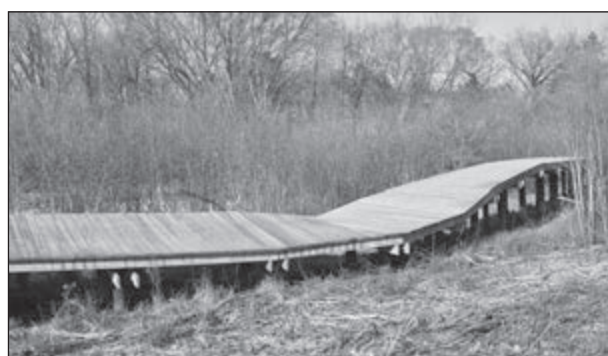
Iola's River Walk needs repair. Emily Conroy Photo
