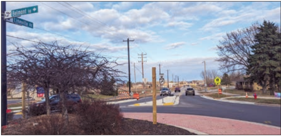
Construction will begin Monday, March 25, on a $9,581,485, two-year project to improve CTH M/Lineville Road in the villages of Howard and Suamico. Staff photo
