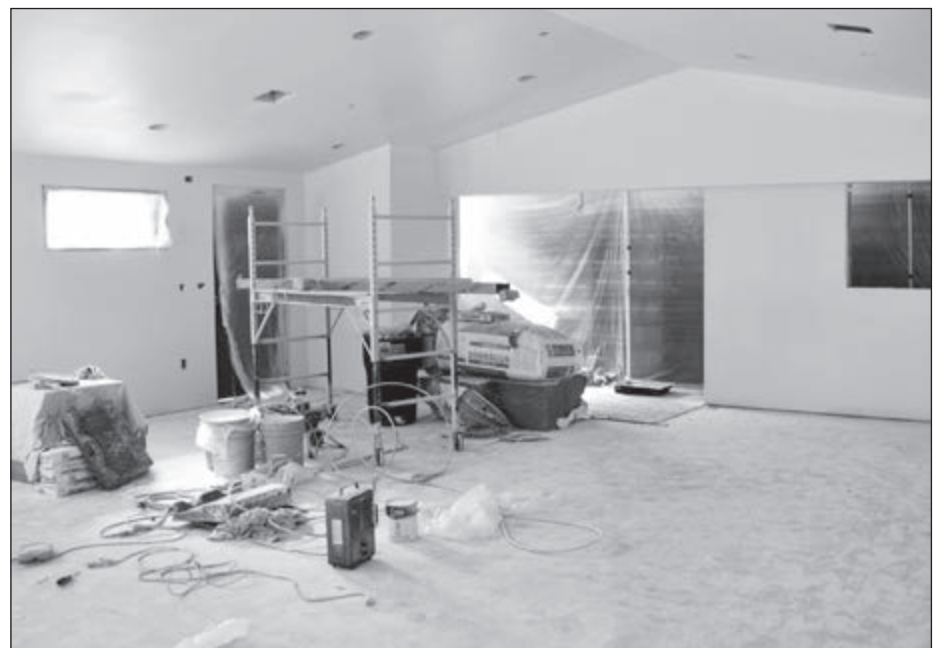
The new addition to the Weyauwega Public Library nears completion. On the interior, there is some painting, flooring and fixture work left. On the Tyvek-covered exterior, siding will be put up soon. Library Director Kelly Kneisler said the project is on track to be finished by late March-early April.
