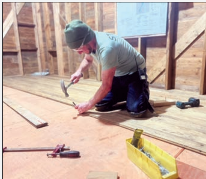
David Haack installs the original flooring. The house was disassembled and transported to Heritage Hill in 18 pieces, including 12 wall sections, four roof sections and two floor sections, where it is being reassembled and prepared for an early May opening. Submitted photo
