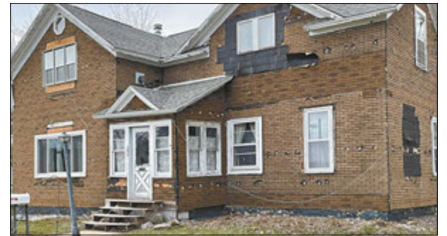
The first layer of siding, containing asbestos, was removed by a specialty company. The Alberts discovered there was another layer of old shingle-style siding on the home that needed to be removed next. Photos courtesy of the Alberts.
