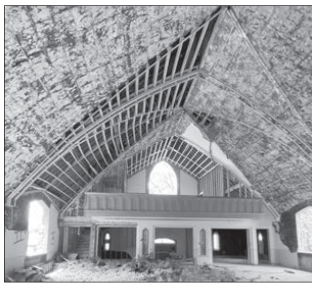
Crews deconstructed the former St. Mary Magdalene's church. Many of the building's features were repurposed or recycled.
