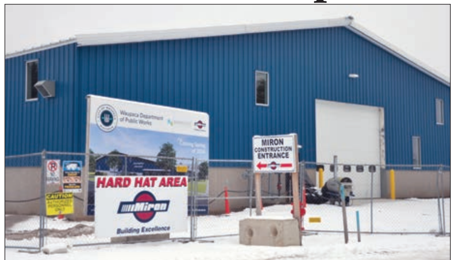
Construction is underway at the city of Waupaca's new Public Works facility.
