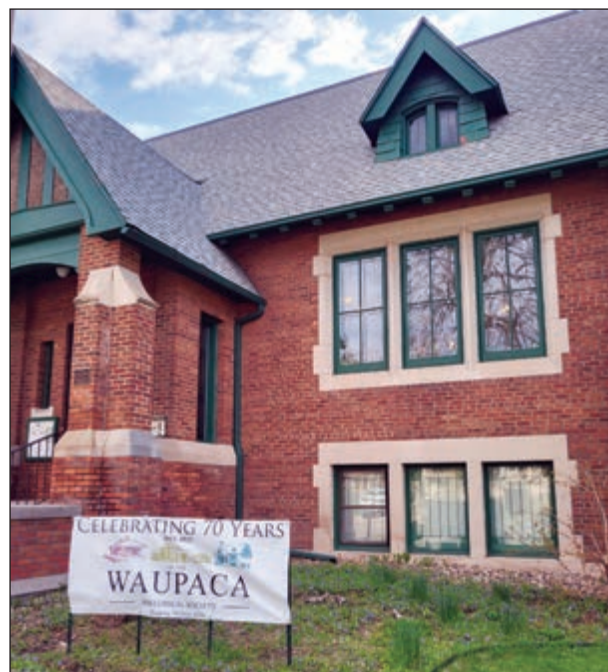
The Holly History and Genealogy Center on South Main Street has a new roof thanks to contributions to the Waupaca Area Historical Society's capital campaign. The society also made other upgrades in the building.
