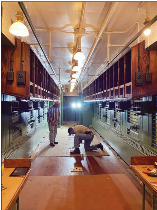
A mix of full time workers and volunteers were tasked with refurbishing the mail slots and overhead bins, refinishing the wood floor and installing new lighting in the car.
