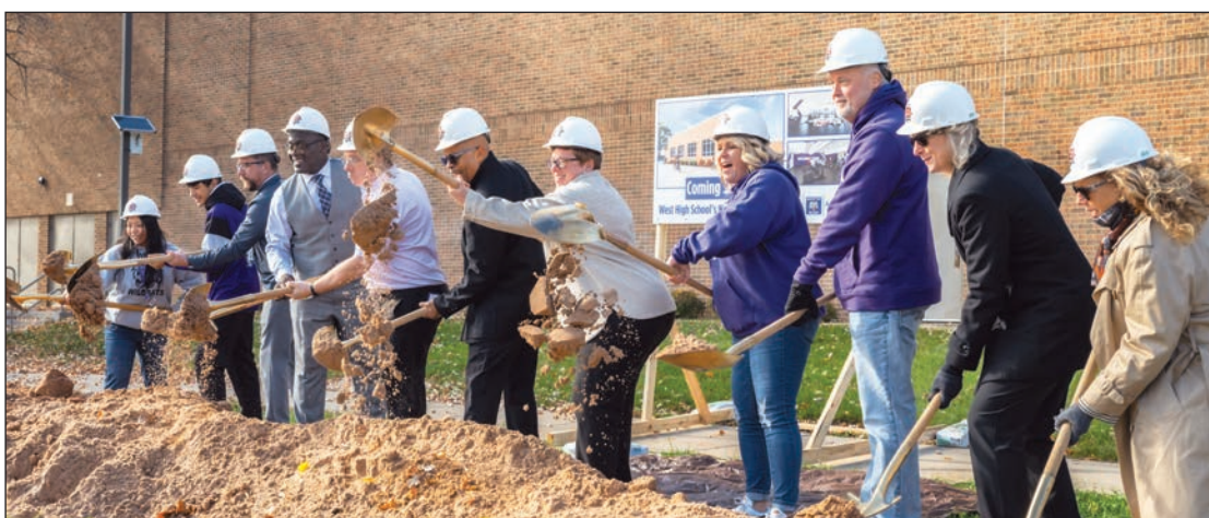
On Wednesday, Nov. 1, Green Bay Area Public School District (GBAPS) and West High School broke ground on an addition to the high school for a new weight room and wrestling space. Shane Fitzsimmons photo
