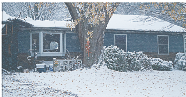
While structurally, most of the home is still standing, the fire, smoke, and water damage is extensive throughout the home. One neighbor's home was also damaged, with the siding on their house melting due to the intense heat of the blaze. Tina L. Scott photo.
