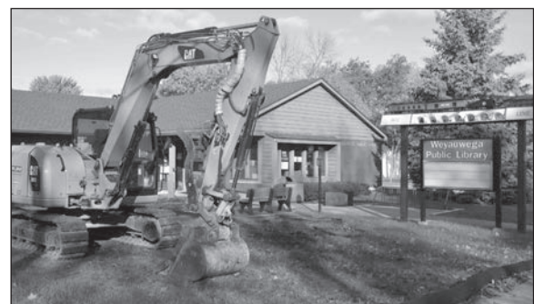
Construction of the new addition at the Weyauwega Public Library has begun and the timeline for completion is targeted for March 2024. James Card Photo
