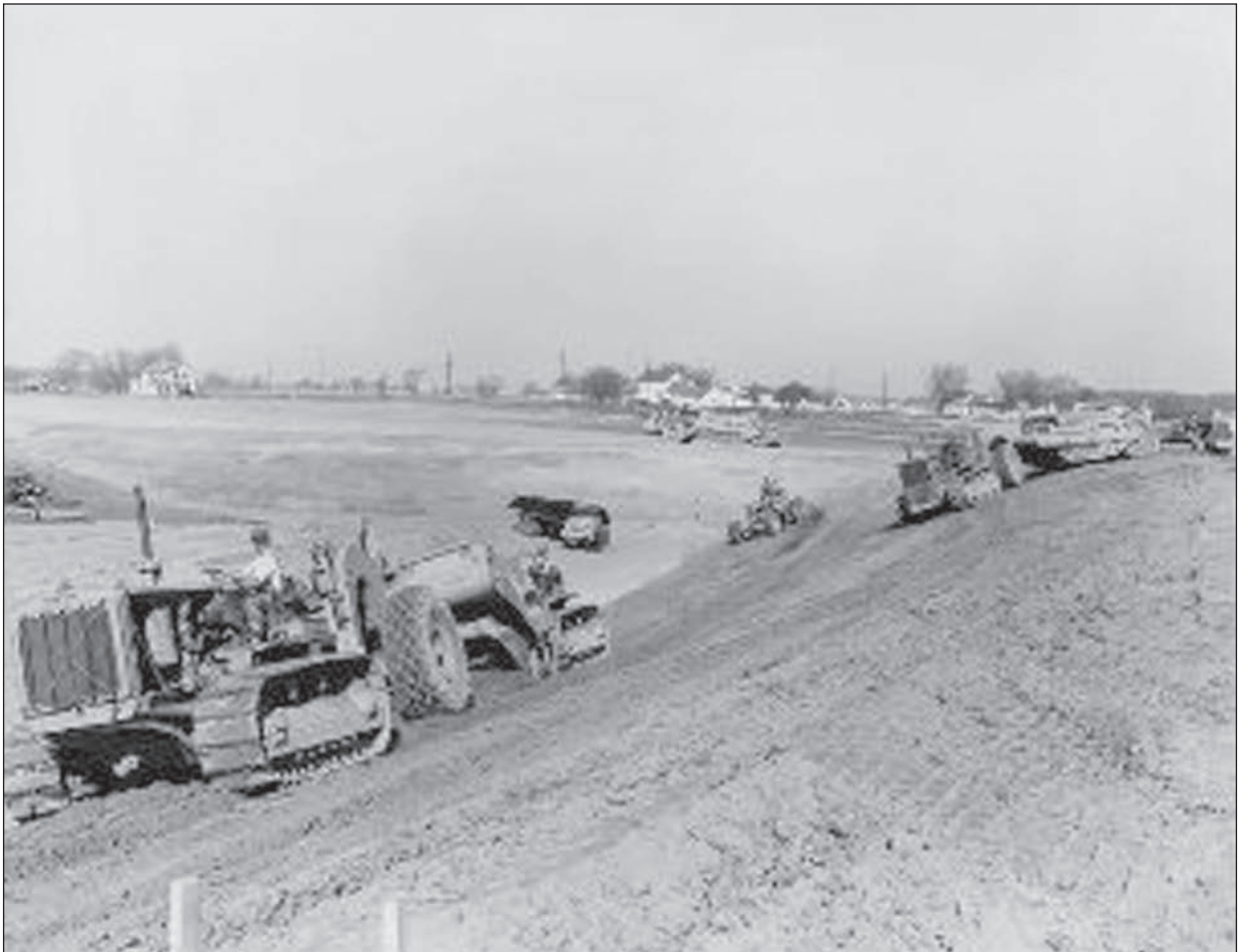
Contractors start to carve out the bowl for the stadium in February 1957.
