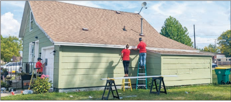
Volunteers work on a home on Chestnut Avenue as part of Good Neighbor Week.
