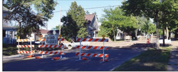
The driving lanes of E. Somo Ave. at N. 6th St. will be temporarily paved ahead of next week's Northwoods Fall Ride.
