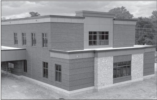
Construction crews are working on the new facility for First State Bank in New London.
