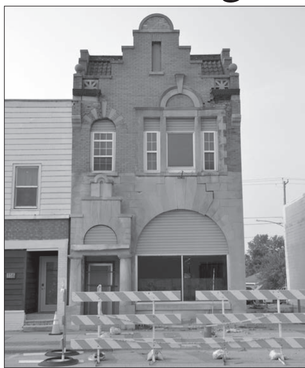
The Weyauwega Common Council voted to raze the building at 118 E. Main St. An architectural report said the building is in danger of "imminent collapse."
