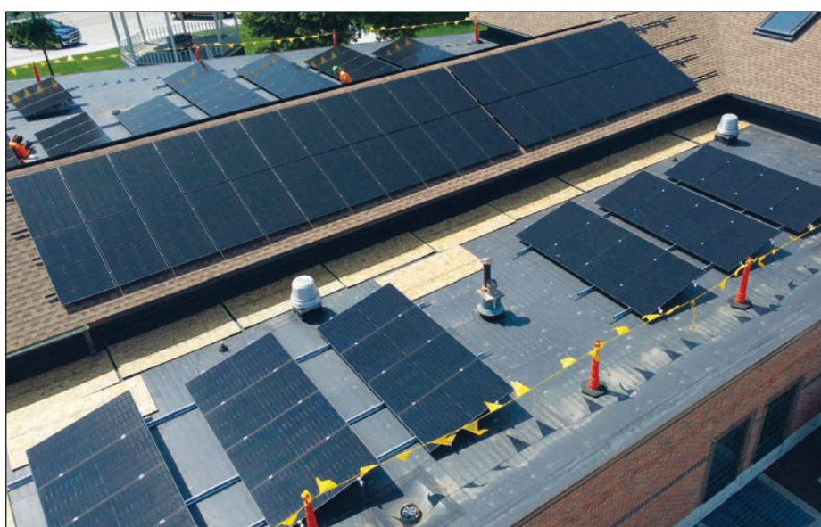
Waupaca has mounted solar panels to the roof of city hall. Submitted Photo
