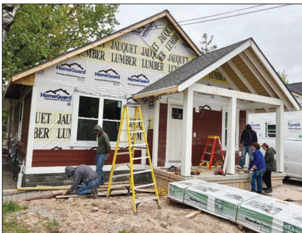
Students working on the siding at the 1208 Doty St. house. Kaity Coisman photos
