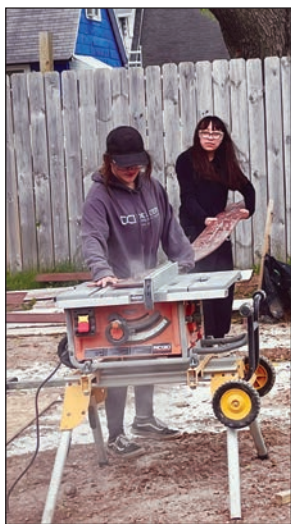
Two Green Bay area students cut siding down for use on the 1208 Doty St. house.
