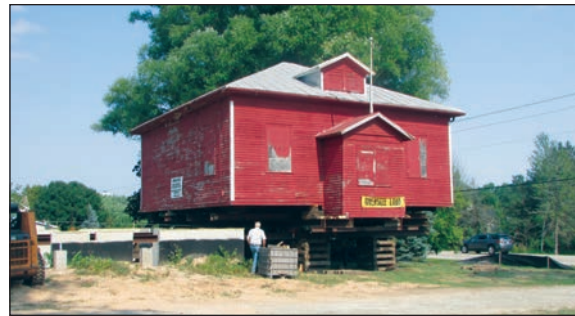
The Tremble School project is focused on renovating the one-room Suamico school that was originally built in 1916 and held classes until 1964; it is the organization’s current biggest project. Submitted photo
