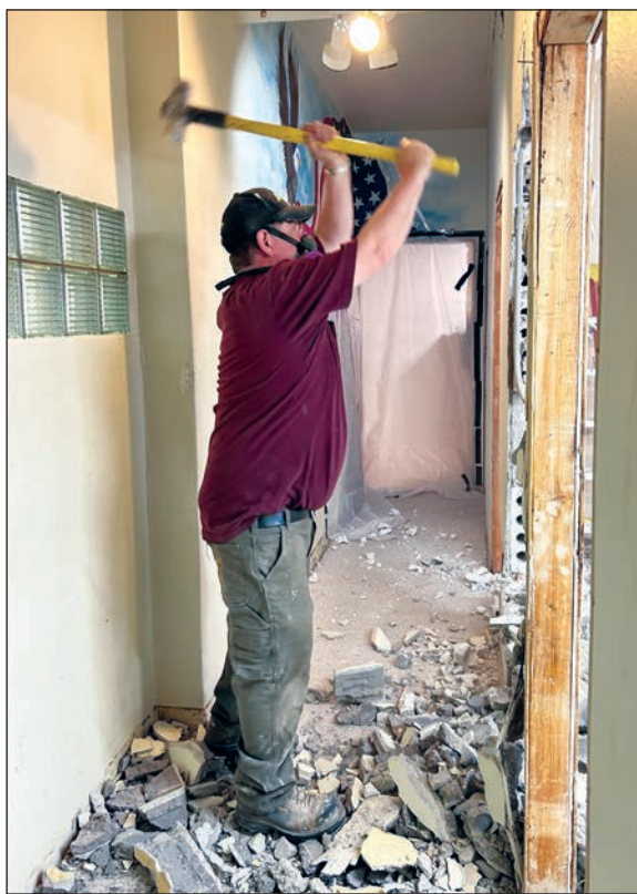
Demolition is well underway at Kilroy's Klub and the Tomahawk American Legion, 327 W. Wisconsin Ave. The team has taken down numerous walls and made some interesting discoveries, including a glass-block wall and a hidden window, which will be repurposed in the remodel. Kilroy's will be open for business again soon, the Legion said. The public is invited to stop by the Legion and check out the progress. To volunteer for one or more of a variety of tasks (excluding construction), contact Tom Pederson, Post 93 Adjutant, at tomahawkpost93@gmail.com. Photos courtesy of Sarah Wolff
