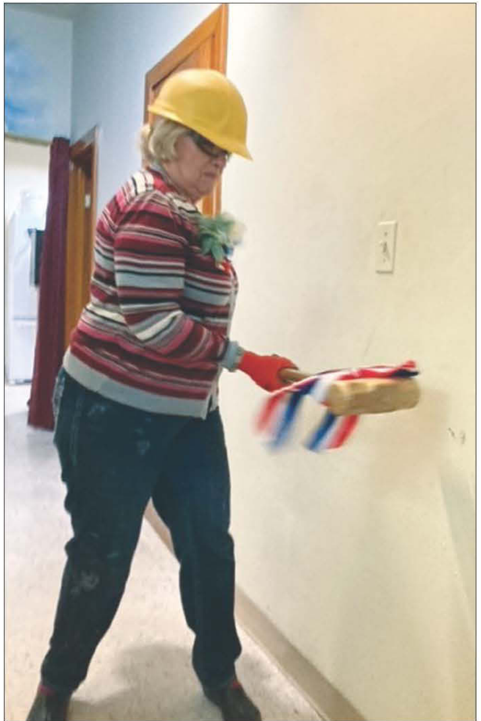
Demolition officially began at American Legion Post 93, 327 W. Wisconsin Ave., Tomahawk, on Thursday, April 20. Jeanie Osero, First Vice President of the Tomahawk American Legion Auxiliary and originator of the building renovation efforts, swung the ceremonial gold sledgehammer to kick off the renovation. Construction will begin soon and is expected to last throughout 2023.
