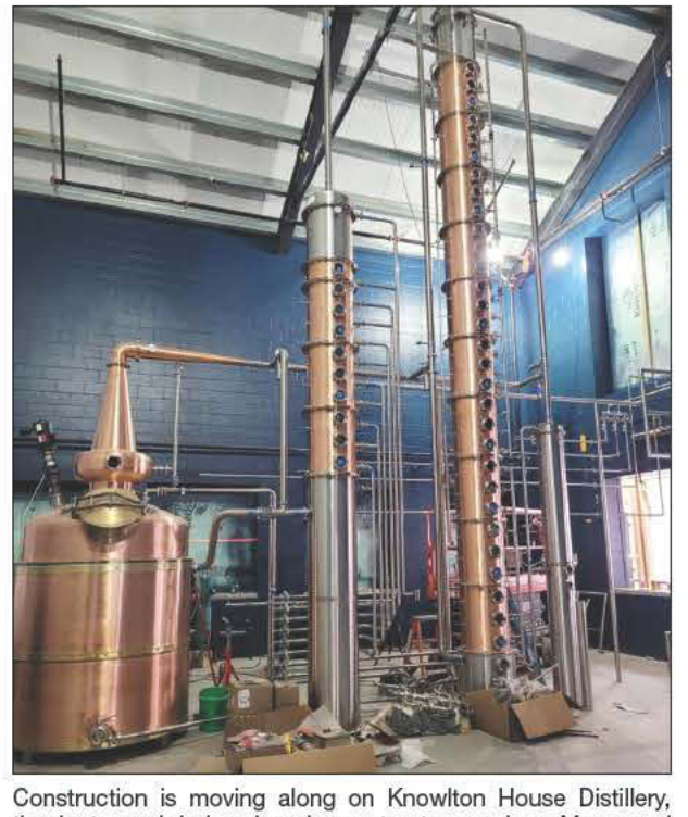
Construction is moving along on Knowlton House Distillery, thanks to work being done by contractors such as Marawood Construction and House of Heating, both of Marshfield. Luke and Heather Mullins anticipate a spring opening. House of Heating photo
