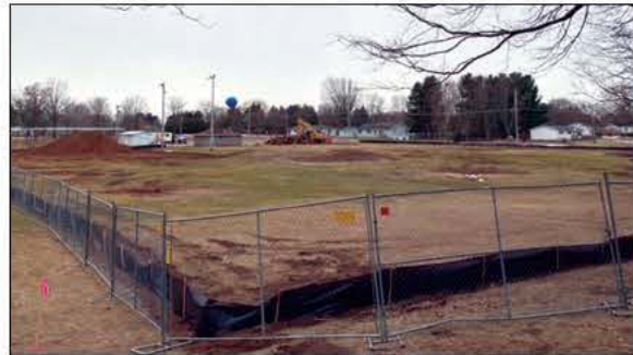
Excavation work and stump removal for the aqua park being built in Clintonville began on Feb. 20. The aqua park project should be completed by the end of July. Photo courtesy city of Clintonville
