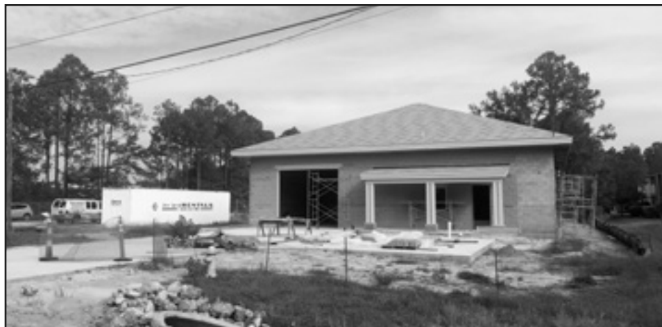
Mayor Bass gave a progress report of construction of Fire Station Number 3 in West Harrison County on Johnson Road. The frame of the fire station's building can now be seen.
