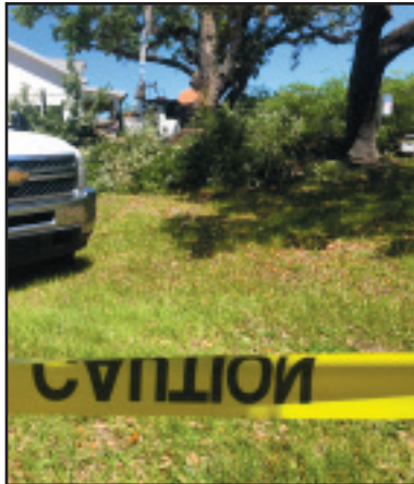
Caution tape sectioned off the site of the tree removal at the corner of 4th Street and Jeff Davis Avenue on April 22.
