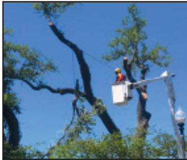
A masked worker begins the task of dismantling, and ultimately, removing a nearly 200-year-old historic oak tree at the corner of 4th Street and Jeff Davis Avenue on April 22.
