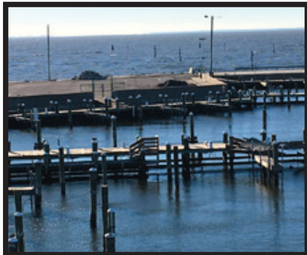
Harbor parking lots and docks also had damage from Hurricane Zeta.
