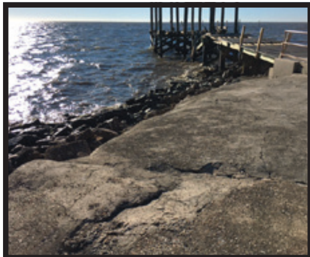
Stringer Pier at Long Beach Harbor after the storm
