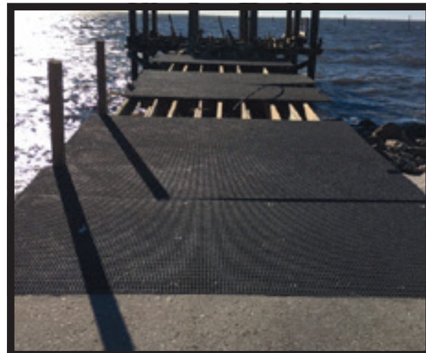
Stringer Pier fiberglass composite decking proved to be a strong successful alternative to wood. Only two sheets detached during the storm. One was located nearby and will be reattached.
