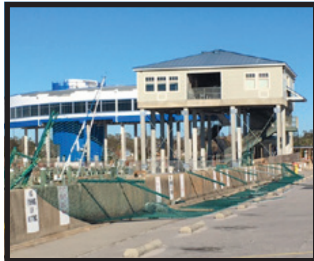
The Harbor fencing sustained significant wind and water damage.
