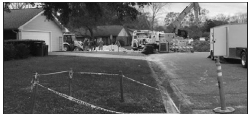
Second sink hole east of Royal Drive on Congress Place.
