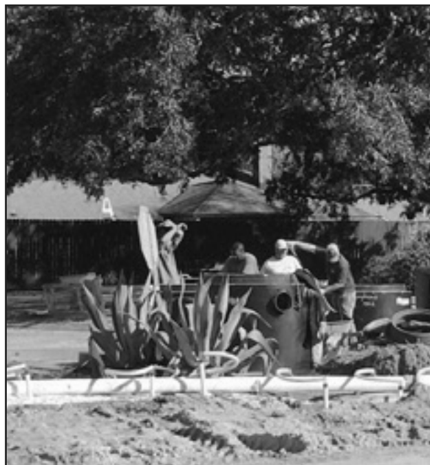
LJ Construction contractors are pictured replacing drain pipes buried ten to fifteen feet along the north end of Royal Drive and the east end of Congress Place.
