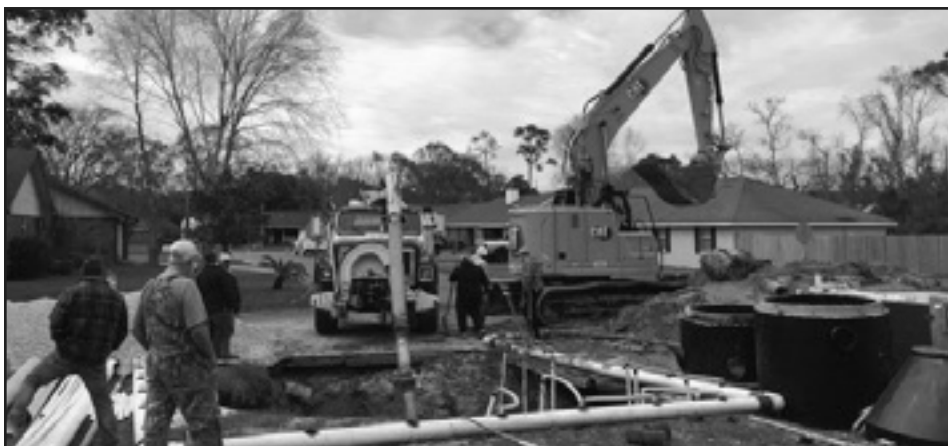
Sink hole repairs being performed on the corner of Royal Drive and Congress Place in Royal Estates.
