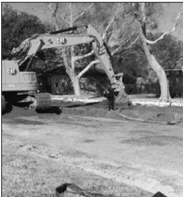
Pictured is the north end of Royal Drive, which was closed for sewer drain line replacement.
