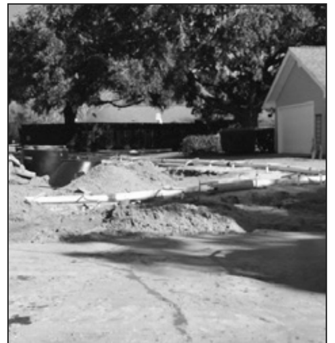
Pictured is the sewer drain line replacement extending down the east end of Congress Place.
