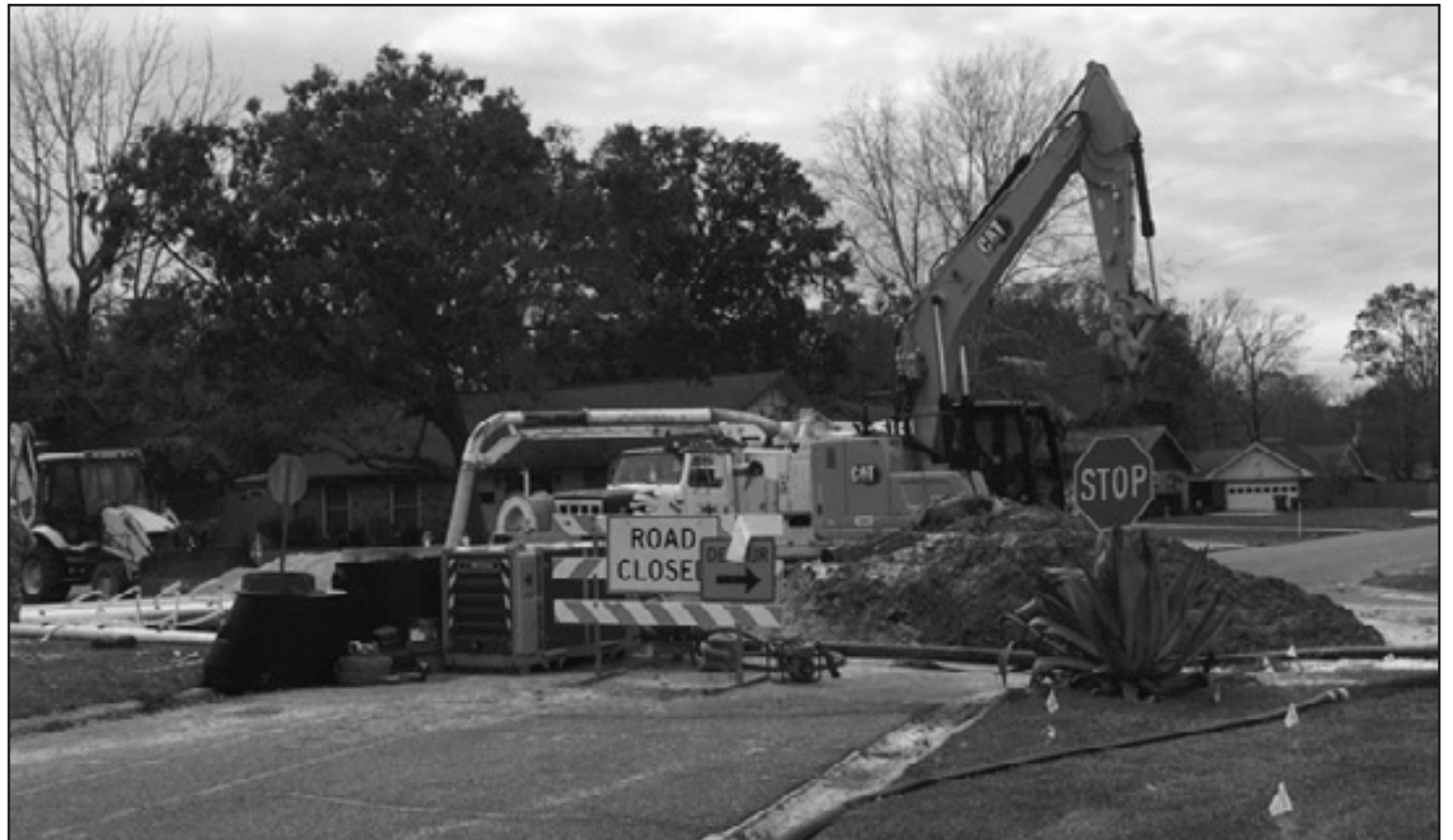
Repairs for two sink holes in Royal Estates started in the late fall of 2021. As the repairs progressed, the contractors uncovered sewage drainage collapsing on the north end of Royal Estates. The City of Long Beach immediately took action to remove and replace the sewage lines on the north end of Royal Drive and Congress Place.
