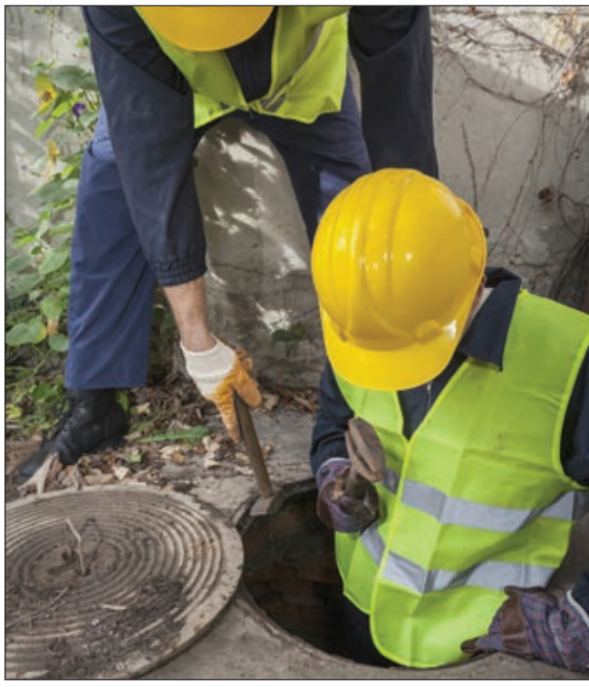
Two young manhole workers, one of them being in the sewer looking for problem to fix.
