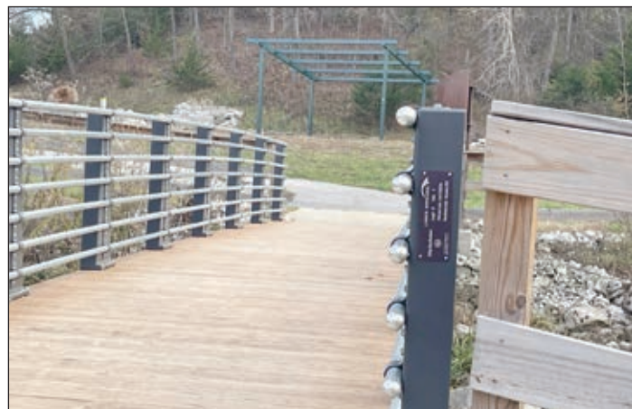
A new pavilion is being erected at the Flats Trail Head on the corner of Missouri and Osteopathy streets.
