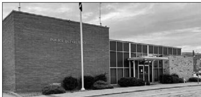
The city's police department is currently housed in a deteriorating former bank building.
