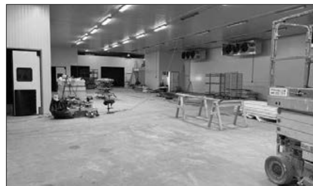
The inside of the new addition to the Western Smokehouse campus in Greentop. The room is awaiting the arrival of two smokers that will be installed inside.
