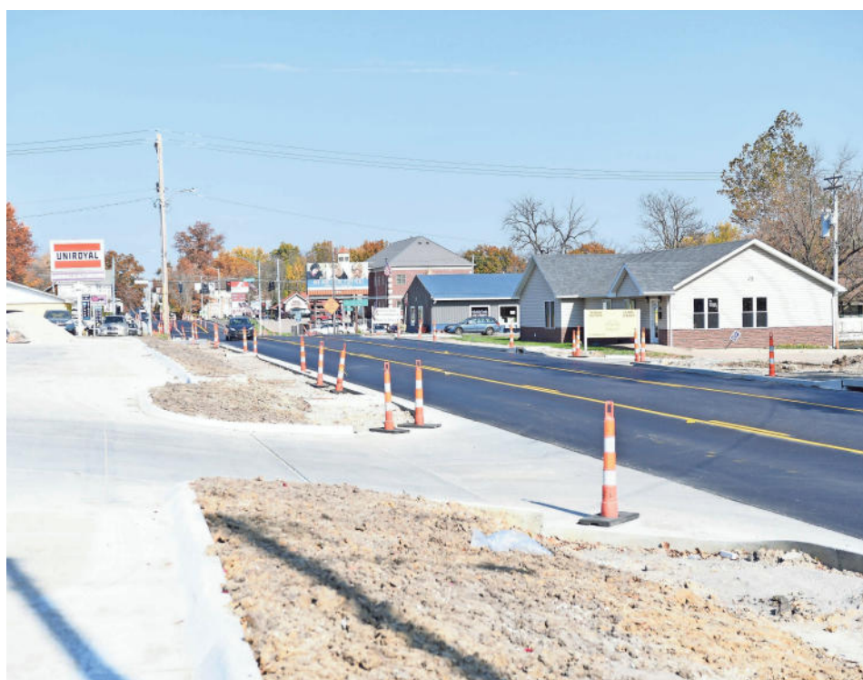
A section of the Better Baltimore Improvement Project, which remodeled a chunk of Baltimore Street in Kirksville. AUSTIN MILLER
