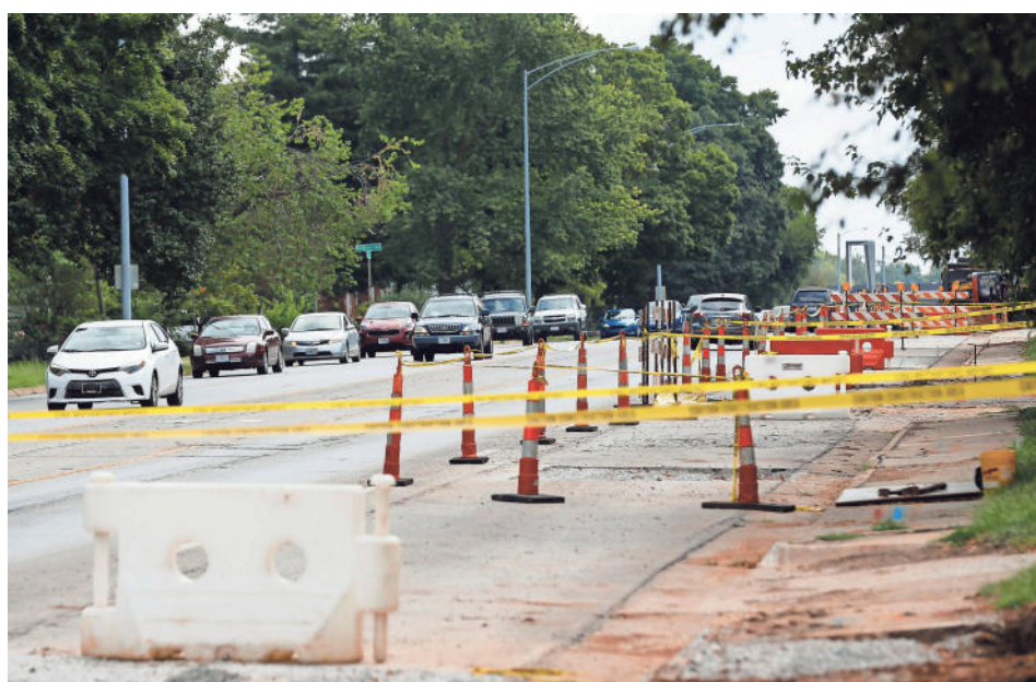
Cars pass by construction on East Sunshine Street on Monday, Aug 16, 2021. City Utilities is replacing the water main in the area and the project is scheduled to be completed by October 1st. NATHAN PAPES/SPRINGFIELD NEWS-LEADER
