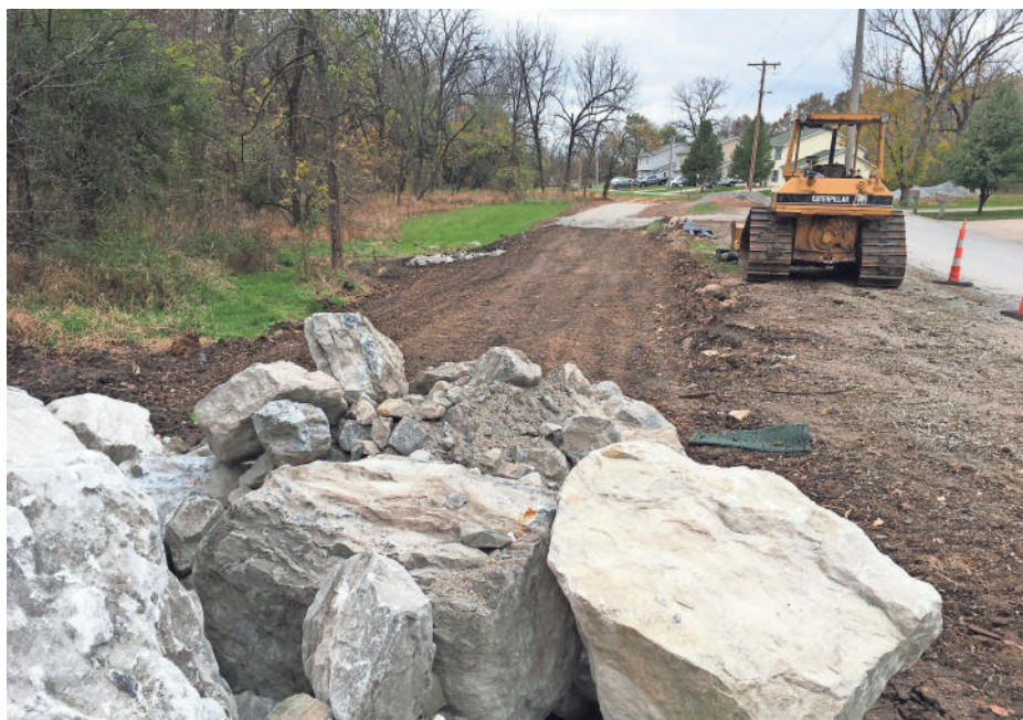
A shot during construction of the Phase 3.1 trail that extends out from the trailhead on Osteopathy. PROVIDED BY ROYCE KALLERUD
