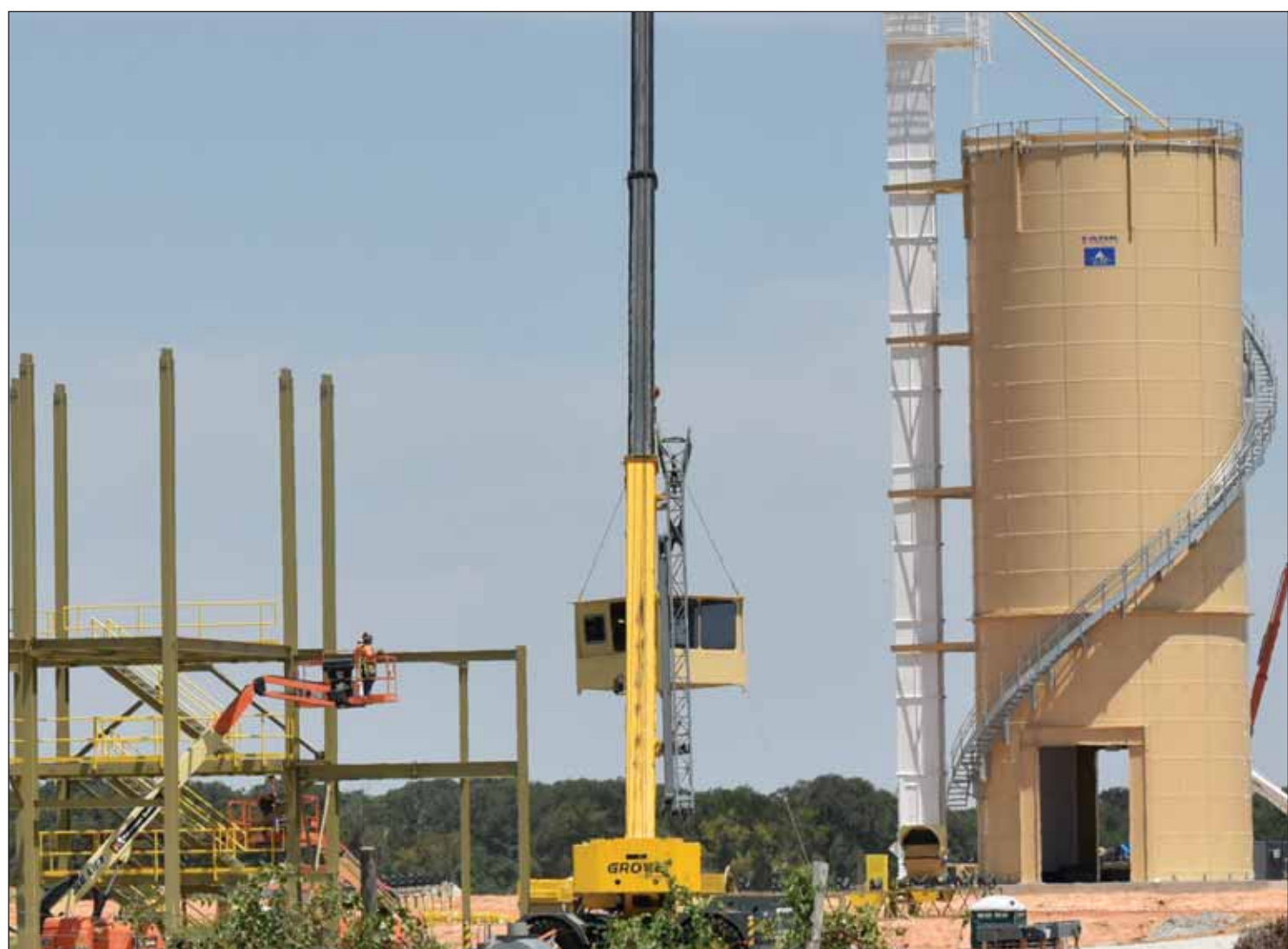
MOVING FORWARD: Construction of the new Vista Sand plant in Tolar is well underway. The plant is located on 500 acres off Electric Road, about one mile east of Tolar. About 60 area residents attended a town hall meeting in January to express opposition to the plant or to ask questions. Vista Sand, which has a plant in the Cresson area, is one of the county's largest employers.
