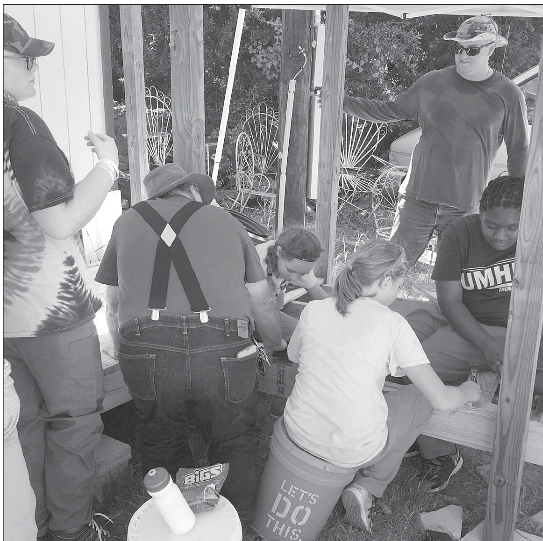
ON A MISSION: Church youth from several churches in Texas served Granbury residents in need through building projects last week. The middle through high schoolers toiled in the afternoon sun, building wheelchair ramps and installing Sheetrock, among many other projects.
