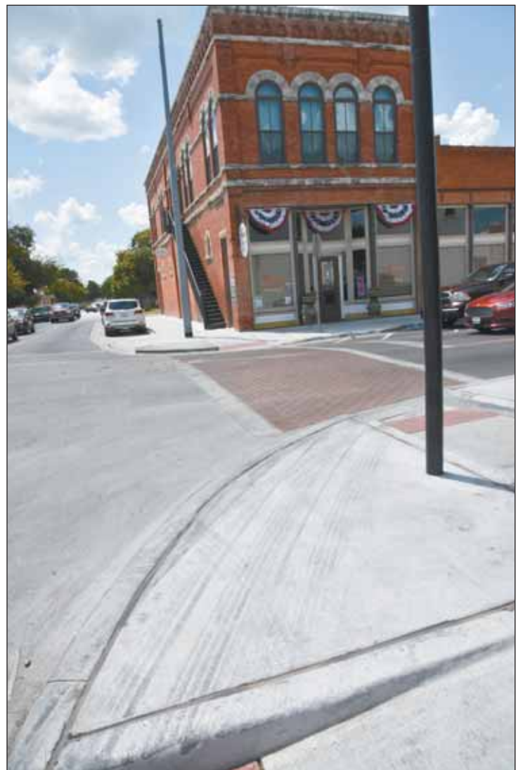
MARY VINSON | HOOD COUNTY NEWS | BUY REPRINTS AT HCNEWS.COM/GALLERIES CUTTING CORNERS: The Downtown Streetscape Project won't be finished until September, but already a problem with turn radiuses has resulted in tire marks on sidewalks and a damaged curb. Some had predicted from the beginning that this would happen, but the City Council hopes to fix the problem.
