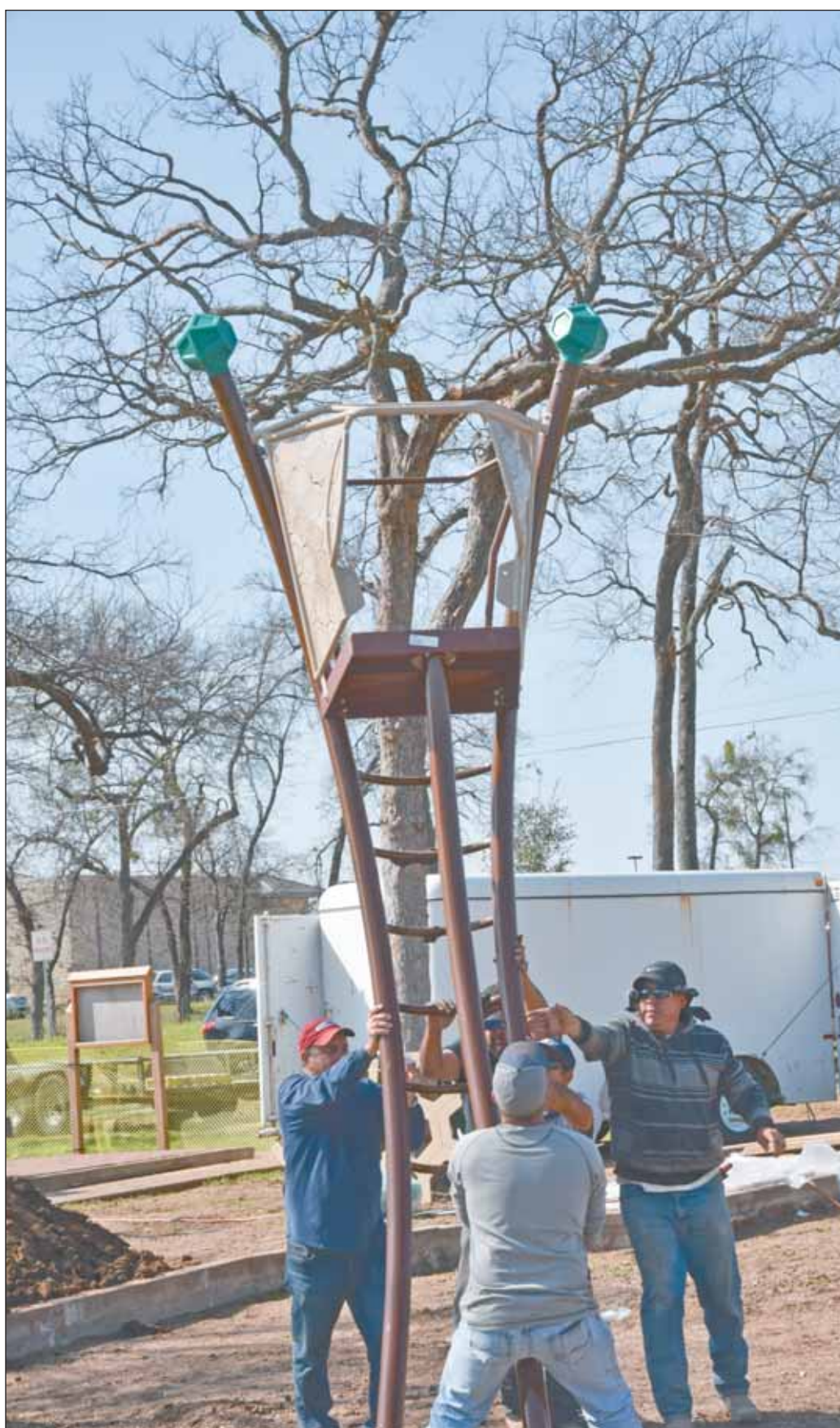
NEW PLAYGROUND: City crews have been busy dismantling the Optimist Playground that has been at the City Park for many years in preparation for installing new play equipment. The $100,000 project is being funded through a gift of $30,000 from the Optimist Club and almost $70,000 from surplus sales tax revenues paid to the city. The new playground is expected to open to the public on March 27, weather permitting.
