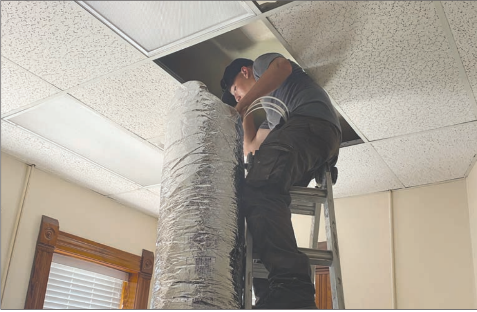
DAVID SCOTT | THE GATESVILLE MESSENGER A worker for Dirty Ducts in Waco installs new ducting in a third-floor office space in the courthouse.
