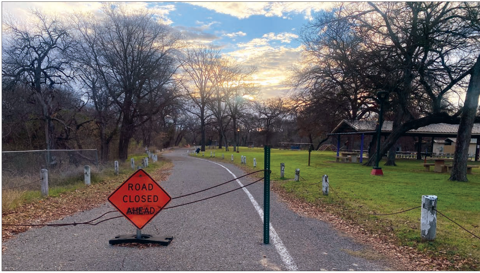
Since 2018, a damaged riverbank at Faunt Le Roy Park has needed repairs.
