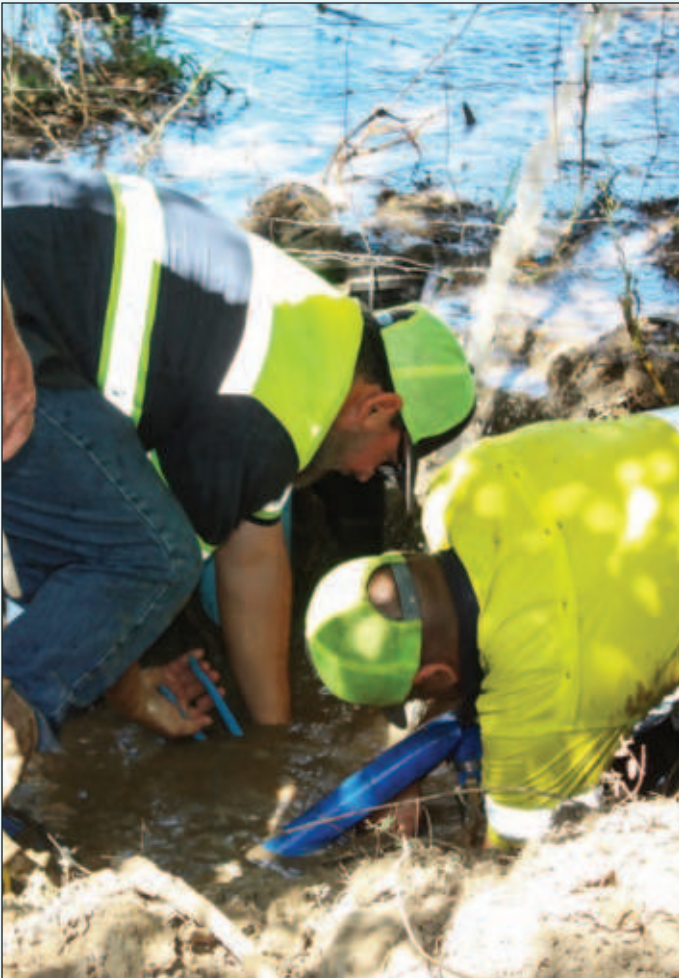
City employees work around the clock to maintain and repair water and wastewater lines.
