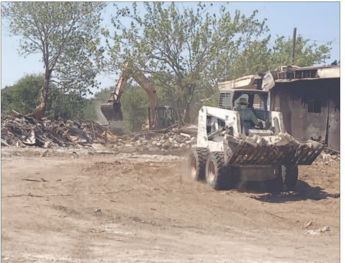
DAVID SCOTT | THE GATESVILLE MESSENGER After years of attempts to have the former Rotunda Nursing Home demolished, action is finally being taken to remove the hazardous structure.
