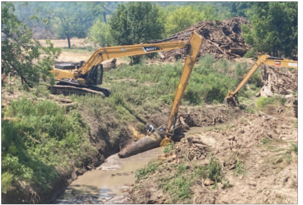
Workers slowly removing massive amounts of timber in the log jam from the Leon River at Mother Neff State Park.
