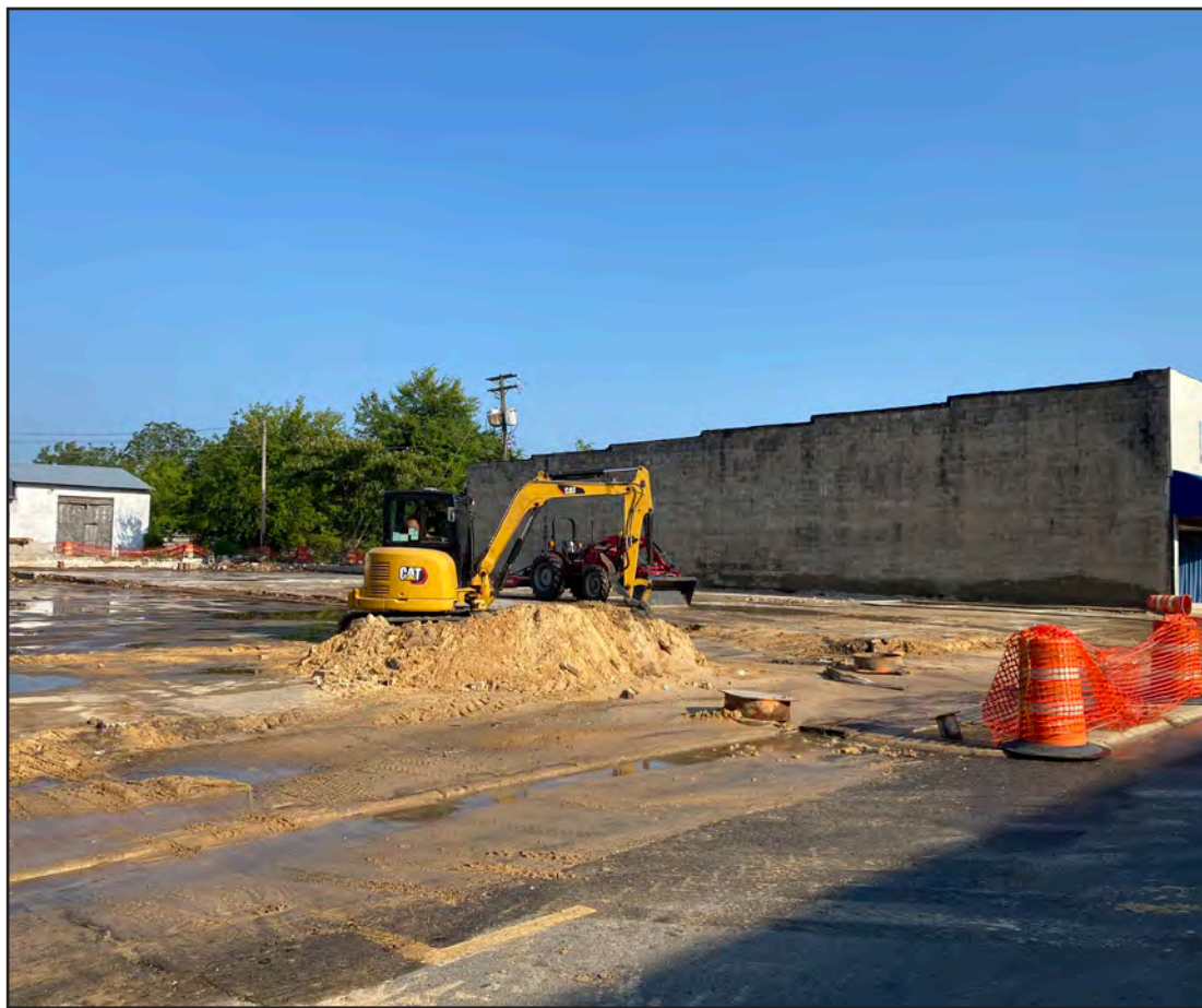
The cleanup at the Bryant Furniture building was completed. The space is now an empty lot. Plans for the lot are still in discussion.
