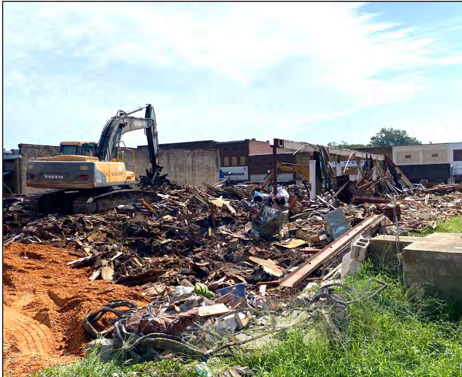
Cleanup has begun at the demolished Bryant Furniture building in downtown Warren. The city was approved to continue the debris cleanup. County crews are hauling off the debris to the county landfill.
