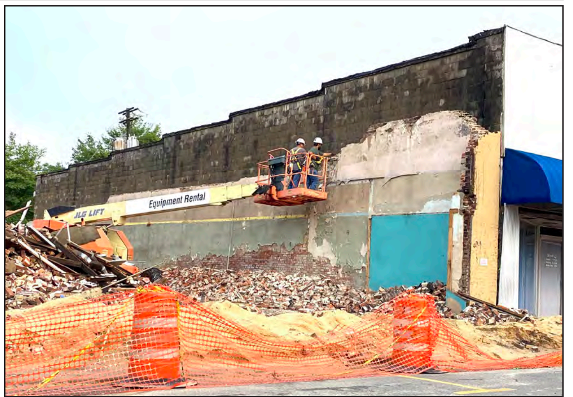
At the city council meeting, the city of Warren was told the wall could be torn down by hand at the Bryant Furniture building until the engineer submits a report. Workers chiseled at the wall by hand.
