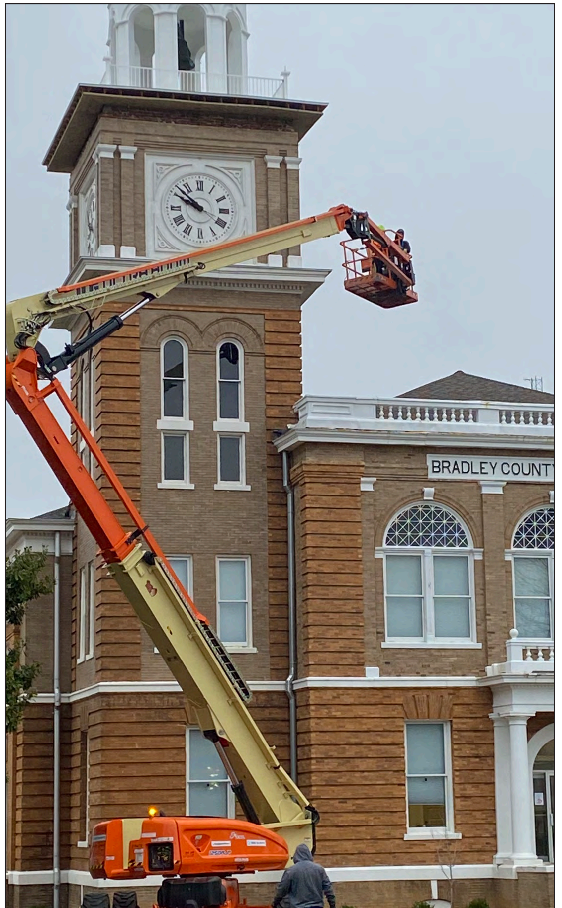
The outside cover of the Bradley County Courthouse is still being worked on as the project gets close to completion.
