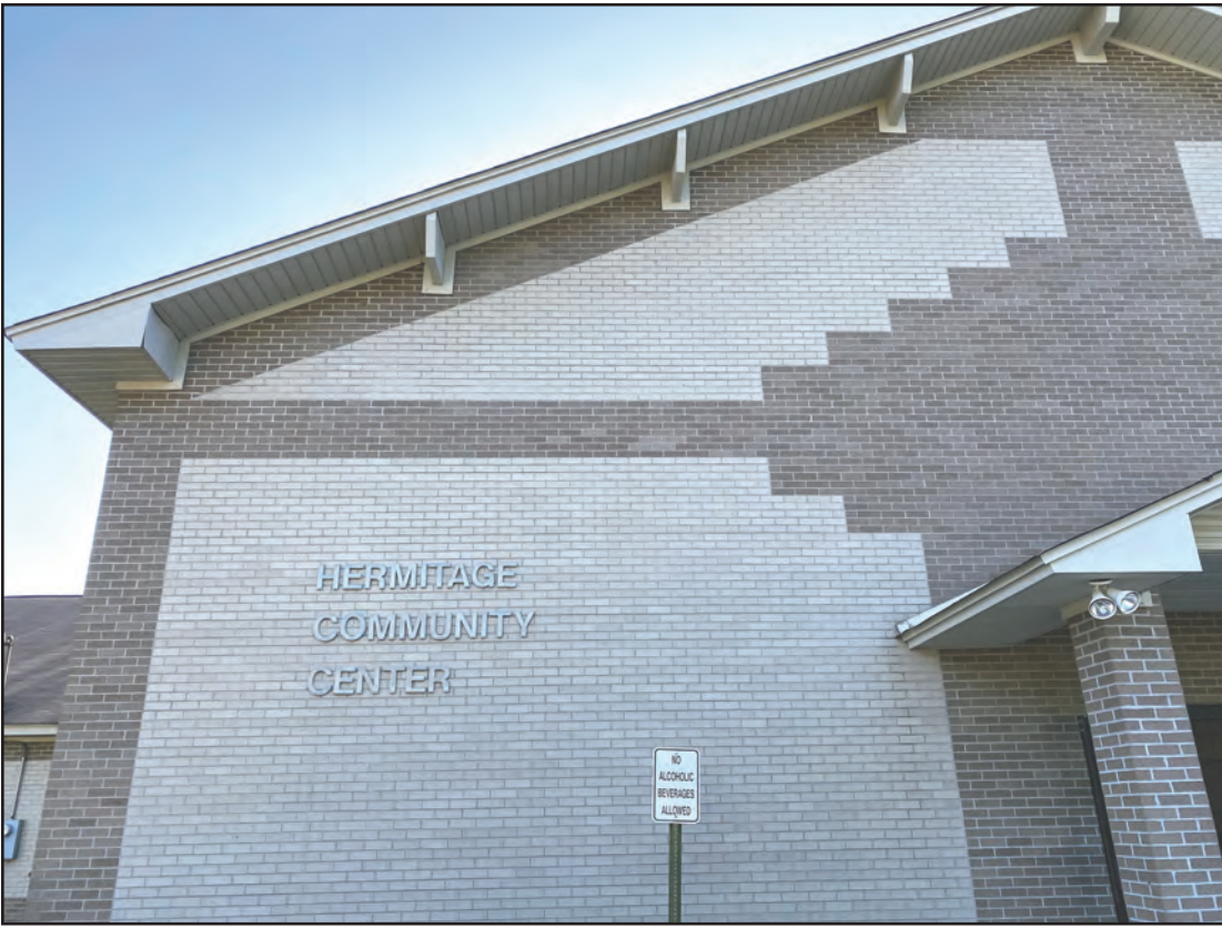
The Hermitage Community Center is in need of roof repairs due to storm damage. The city will assess the damaged to determine the cost.
